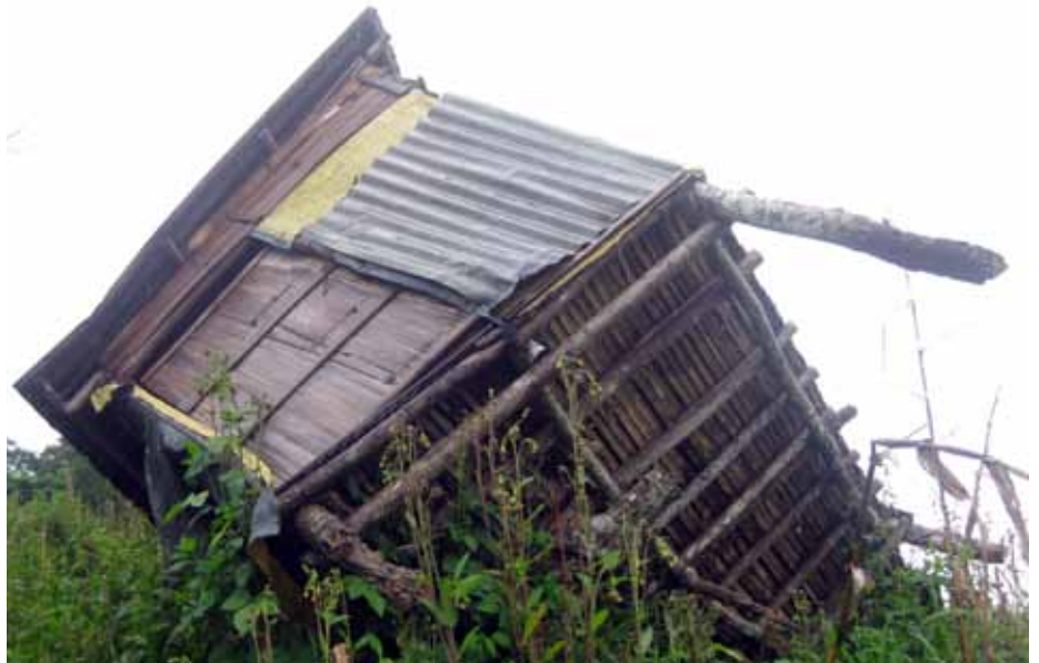
CC PADATA | Destroyed house of a PADATA member.
